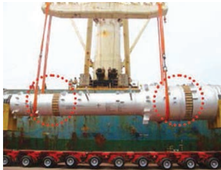
A single crane lifts a column horizontally. The position of the slings here, offset from wooden battens, indicate an off-centre CoG.
