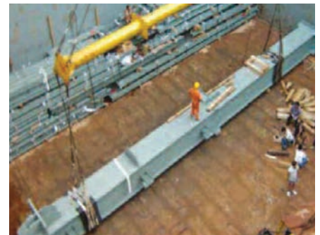
Well-stowed structural steel (athwartships direction) in the hold bulkhead
