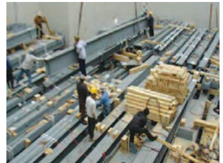
Well-stowed structural steel (fore and aft direction), with adequate dunnage between tiers
