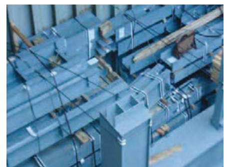
Bundles of prefabricated structural steel on the top tier adequately secured with wooden chocking and wire rope lashings
